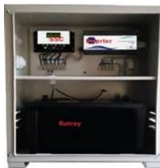
Gambar 13 Panel Box listrik Hybrid
