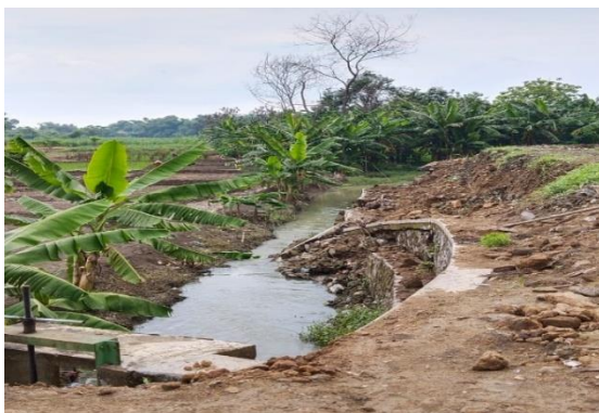
Figure 4. The Banyulegi Village embankment collapsed due to flooding from the Lamong River in 2022
