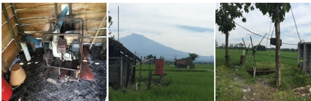
Picture 3. Diesel pump in 30m depth well, many hut in rice field for well equipment, and deep well using electric submersible pump in rice field area
